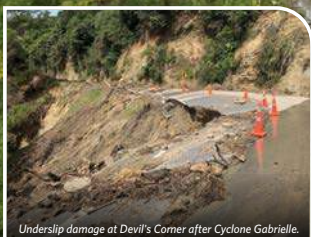
Underslip damage at Devil's Corner after Cyclone Gabrielle.
